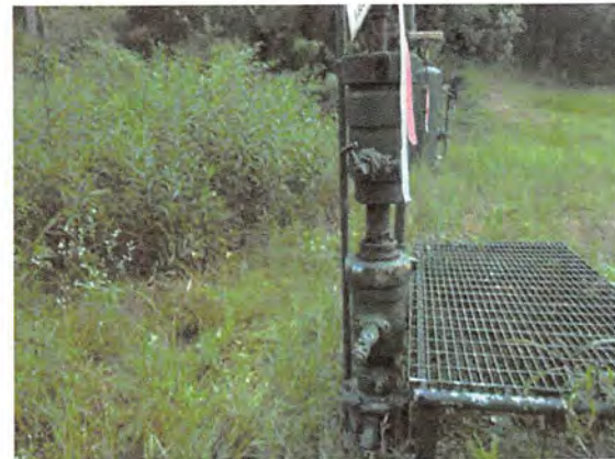
WV 151281 McKinley #8184 Wellhead
