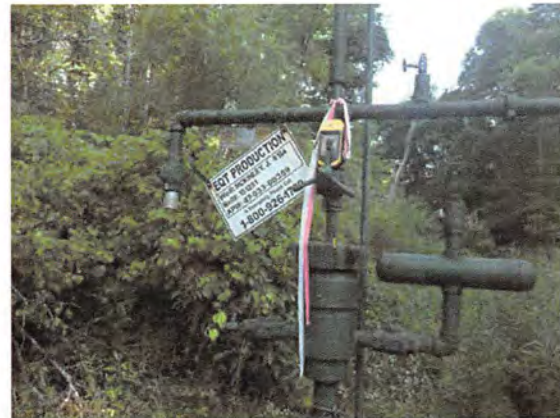
WV 151281 McKinley #8184 Wellhead
