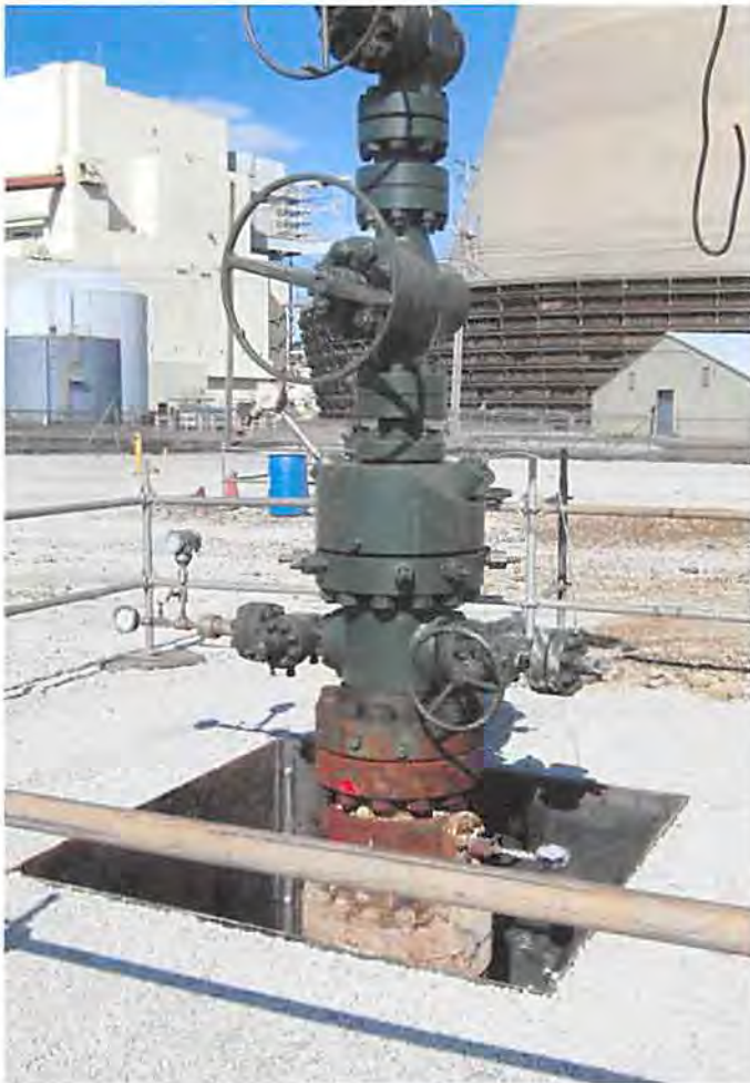
Figure 4: AEP-2 Wellhead and Christmas Tree, above grade components
