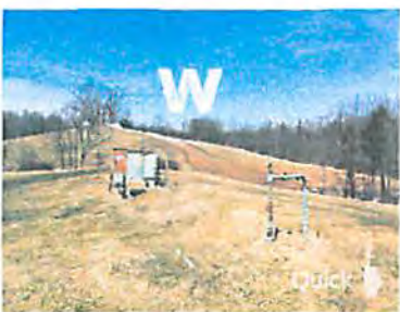
◇ EXISTING GAS WELL EQUIPMENT
