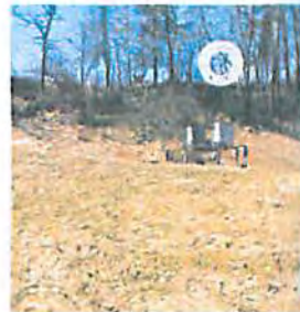
◊ EXISTING PIPELINE METERS & PIG LAUNCHERS
