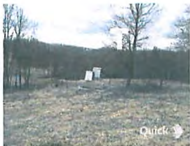
Ⓣ EXISTING PIPELINE METERS & PIG LAUNCHERS
